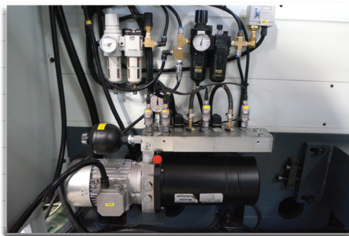
Hydraulic power unit
